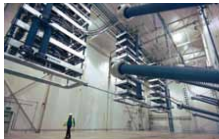
Thyristor blocks for HVDC transmission
