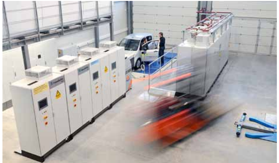
Testing Centre for electromobility and battery converters
