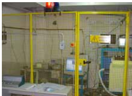
Fig. 1 – The high voltage test room.
