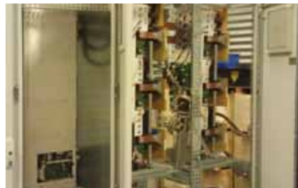
1 MVA power stack. IGBT modules.
