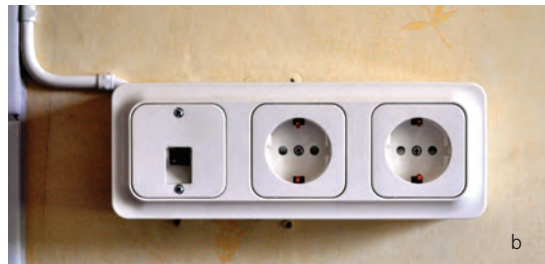
b) The housing on the wall with two electrical outlets and one RJ45 outlet (with an O/E converter behind it). The visible electrical cable is a "home installation" connecting to another electrical outlet. The "real" electrical cabling is hidden behind the walls but visible through the housing in a).
