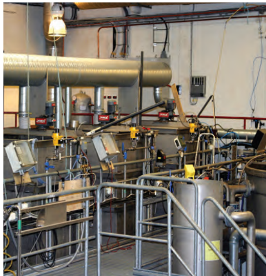
The test facility at the wastewater treatment plant at Hammarby Sjöstad.
