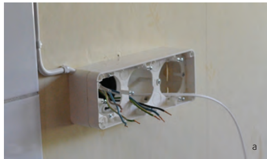
a) The new partly homemade box on the wall replacing the old box on the table. The POF cable is seen to the right.
