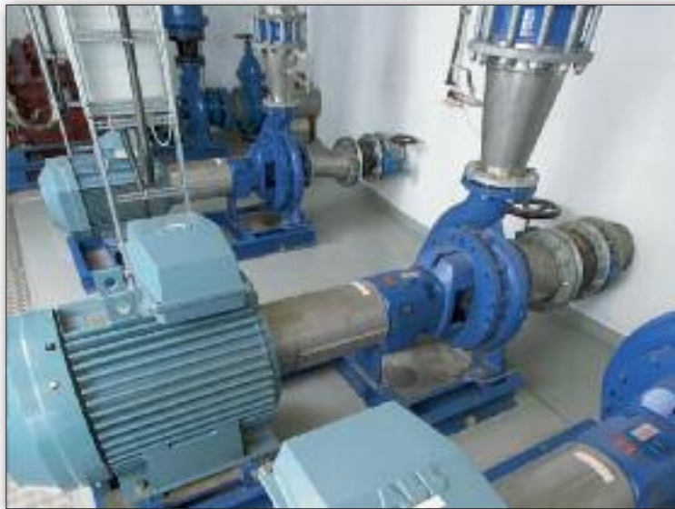
Fig. 4: The pressure boosting station in Pietarsaari's water utility 12 . Copyright © ABB. All rights reserved.
